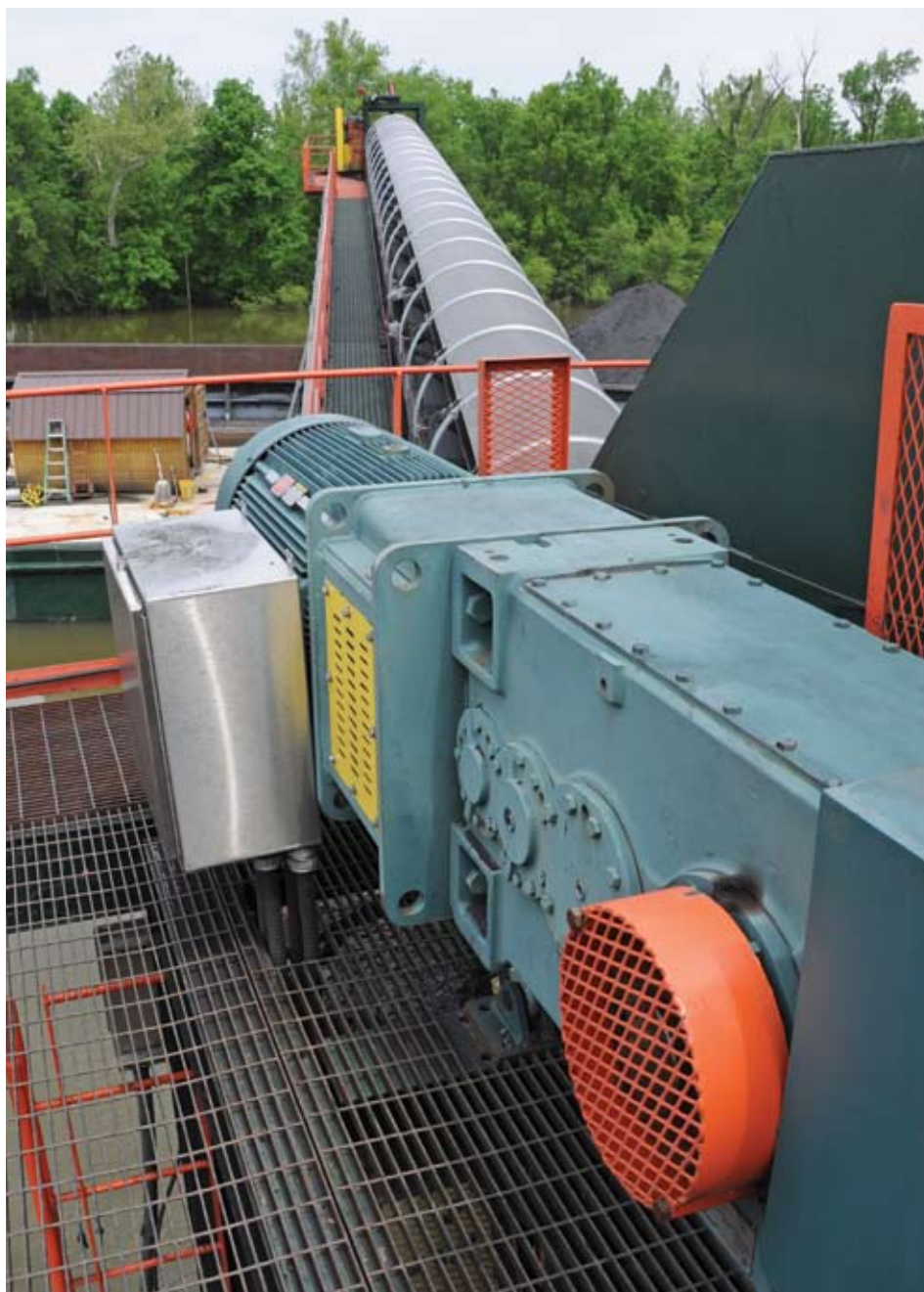
This 285K MagnaGear XTR reducer and 350 HP Mining Industry motor powers the 3,950-foot-long conveyor that carries coal from the mine site to the river barge. Coal is transported 45 minutes up the Green River to the Armstrong Coal dock at its prep plant.
