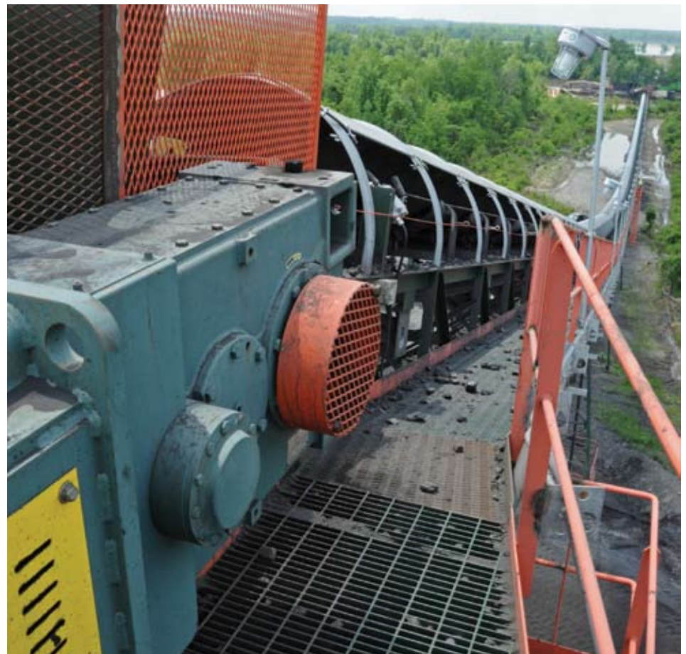
A 210K MagnaGear XTR was selected to operate this 1,197-foot-long conveyor, with an 86-foot lift. This conveyor moves coal from the river barge to Armstrong's prep plant.
